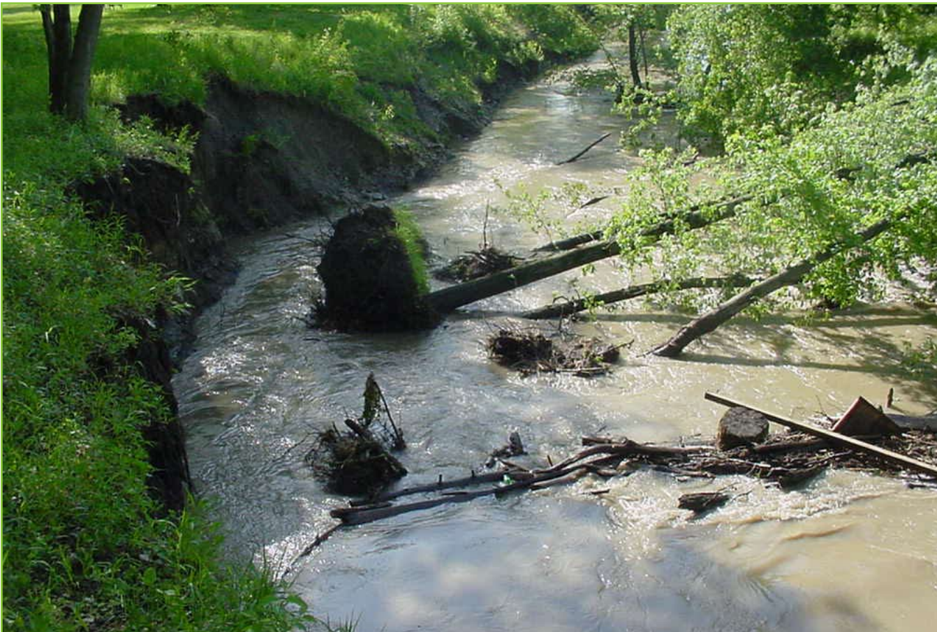
This stream is experiencing extensive erosion. Improved storm water management by Parkville and surrounding jurisdictions will help minimize degradation to streams and preserve their health and water quality.
